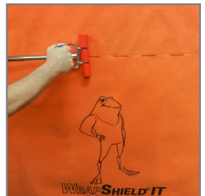
11. Immediately roll the integrated tape horizontal seams with floor roller to ensure full contact.
