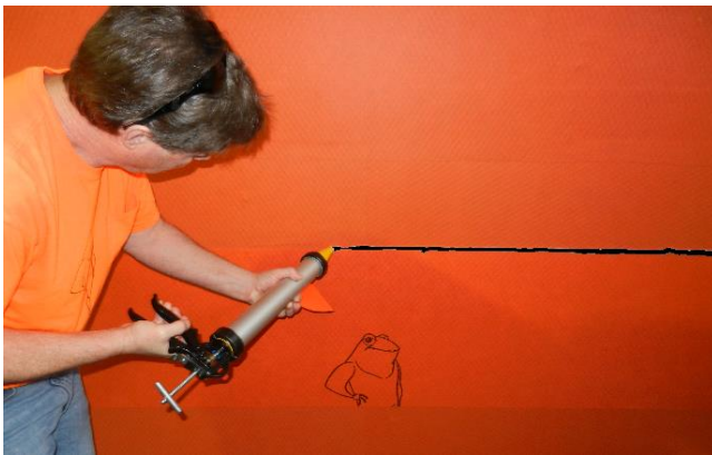
Apply 3/8" (9.5mm) minimum bead line of VaproBond to the reverse lapped membrane.
