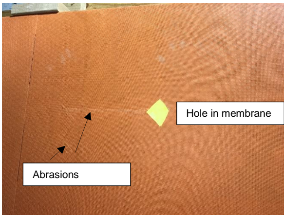
Membrane abrasion and/or hole, prior to repair.
