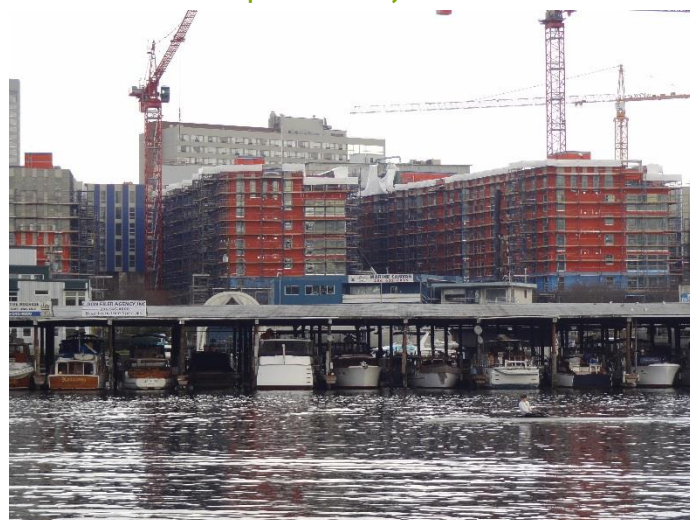
Over 400,000 sq.ft. of WrapShield Water Resistive Vapor Permeable Air Barrier Membrane was installed on Mercer Court Apartments.
