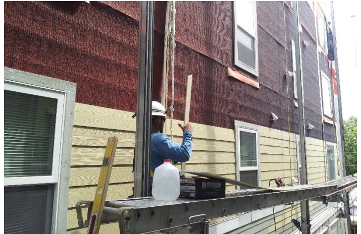
Over 5,000 sq. ft. of WrapShield RS Rain Screen Water Resistive Vapor Permeable Air Barrier Sheet was installed at Two Twenty Apartments in Seattle, WA.
