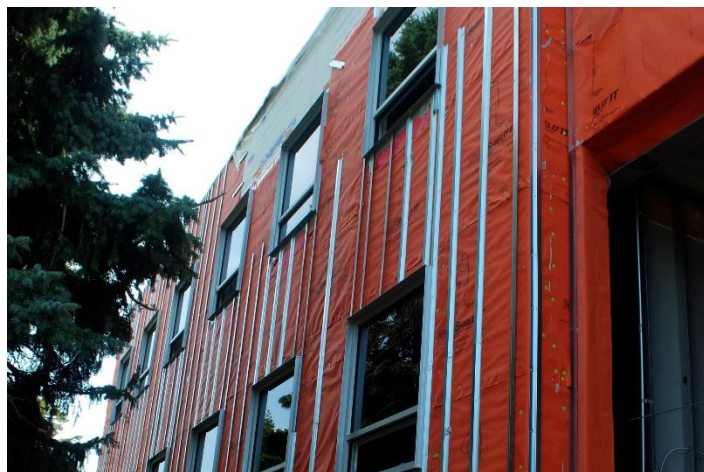
Over 5,000 sq. ft. of WrapShield was installed on Twin Cities German Immersion School in St. Paul, MN.
