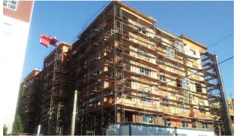
Over 280,000 sq. ft. of WrapShield Water Resistive, Vapor Permeable Air Barrier Sheet was installed on the True North apartment complex located in Seattle, Washington.
