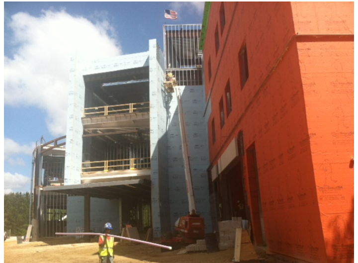
WrapShield SA Self-Adhered Water Resistive Vapor Permeable Air Barrier Sheet was installed.
