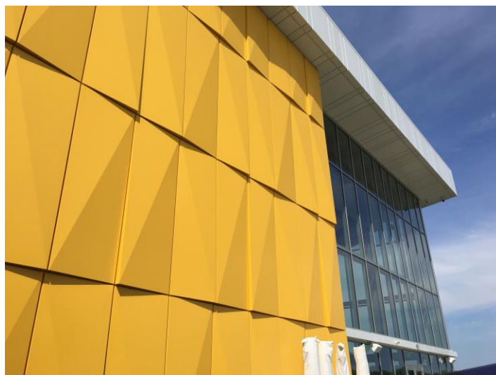
WrapShield SA Self-Adhered was installed behind Alucobond panels by the pool area of the resort.
