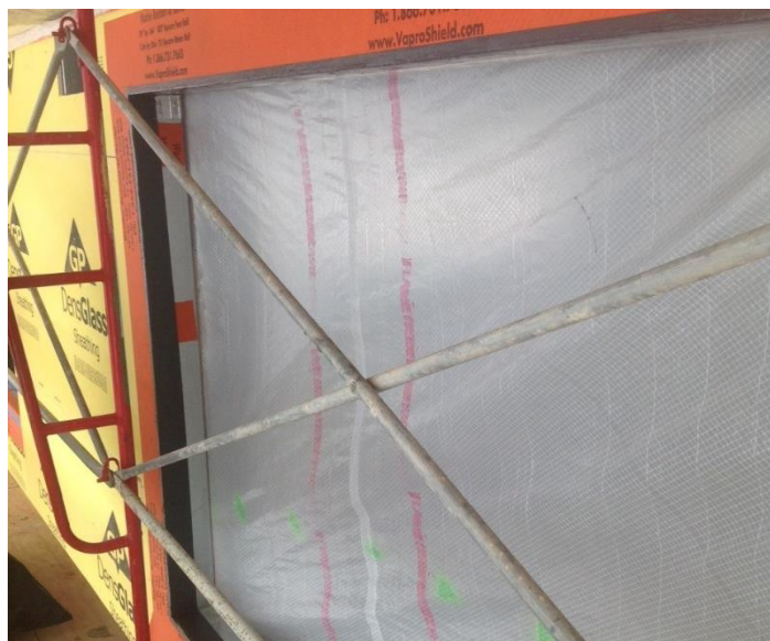
VaproLiquiFlash was used as a liquid applied waterproof flashing material for window and door interfaces.
