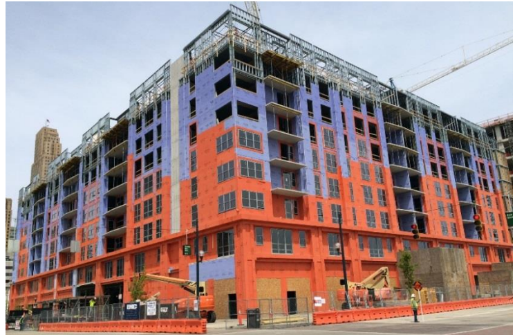
150,000 sq. ft. of WrapShield SA Self-Adhered Water Resistive Vapor Permeable Air Barrier Sheet was installed on the Radius at the Banks Mixed-Use Building.
