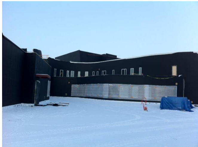
Two layers of WallShield Black Water Resistive Barrier Sheet was installed on the Tanana Chiefs Clinic.
