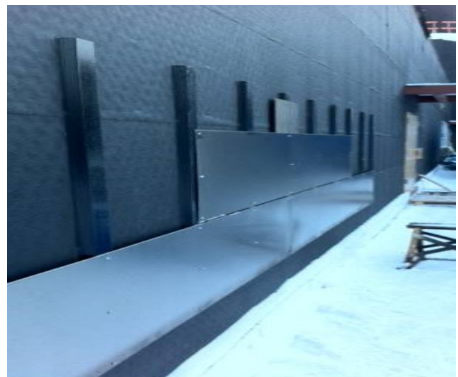
Two layers of WallShield Black were installed behind phenolic and stainless steel metal panels.
