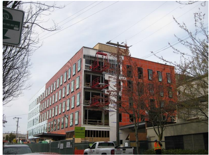
Over 30,000 sq.ft. of WrapShield Water Resistive Vapor Permeable Air Barrier Membrane was installed on the Swedish Ballard Hospital.
