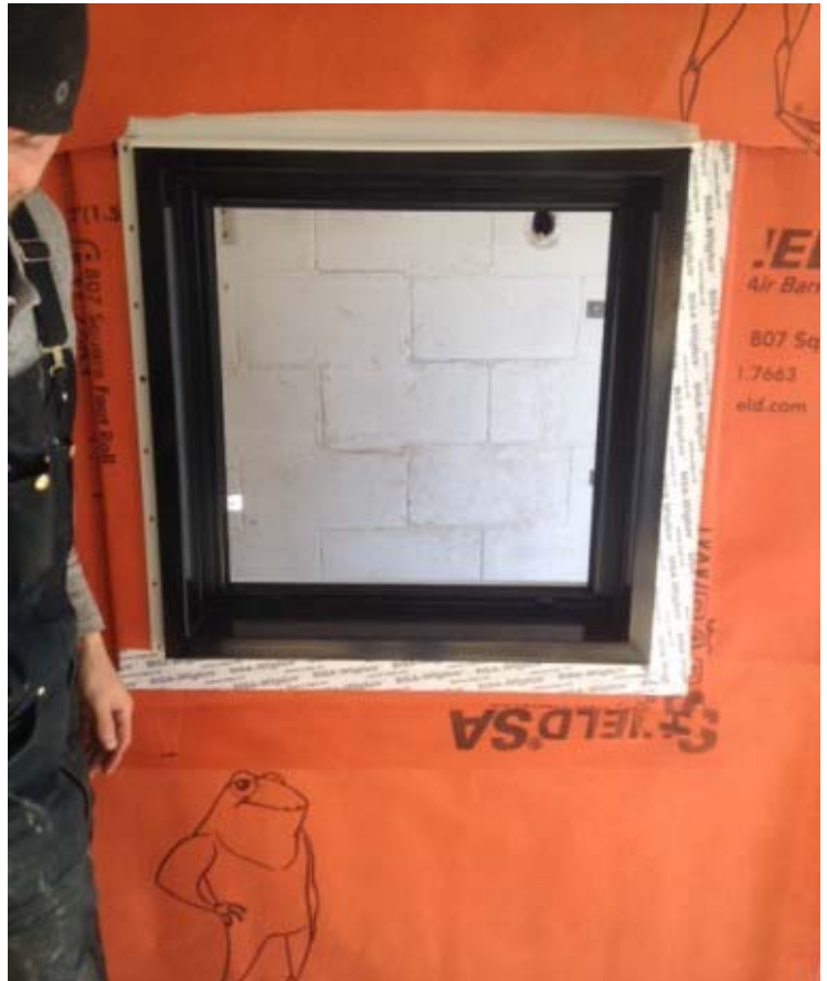
To fix the competitor system's failure, over 2,000 sq. ft. (185.81 M 2 ) of WrapShield and VaproLiqui-Flash were installed as a retrofit on a south end home located in Halifax, Nova Scotia.
