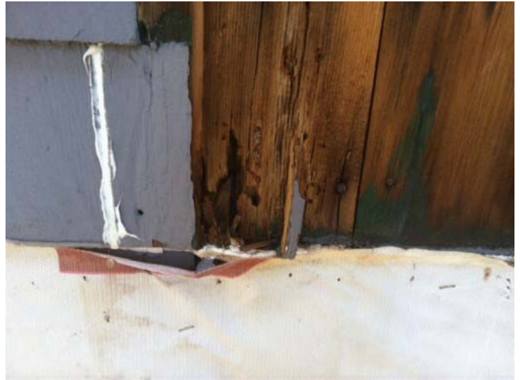
The previous contractors applied a competitor housewrap and tape to seal the joints. Without proper flashing, the installation left incoming water no where to go. This caused extreme water damage and rot. The problem was solved with WrapShield which can protect your building from the damaging effects of moisture intrusion and entrapment
