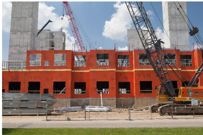
WrapShield SA Self-Adhered WRB/Air Barrier panels (orange) are being installed on the Skyvue Apartments in Lansing, MI.
