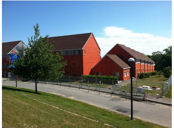
WrapShield SA Self-Adhered Water Resistive Vapor Permeable Air Barrier Sheet was installed on the renovation of the dormitory.
