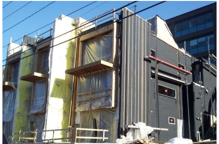
72,000 sq. ft. of RevealShield SA Self-Adhered Water Resistant Vapor Permeable Air Barrier Membrane (black) was installed at The Residences at Fairview in Seattle, WA.
