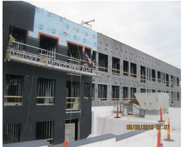
Over 20,000 sq.ft. of RevealShield UV Stable Water Resistive Vapor Permeable Air Barrier Membrane was installed on the Woodward Gardens Apartment Complex in Detroit, MI.
