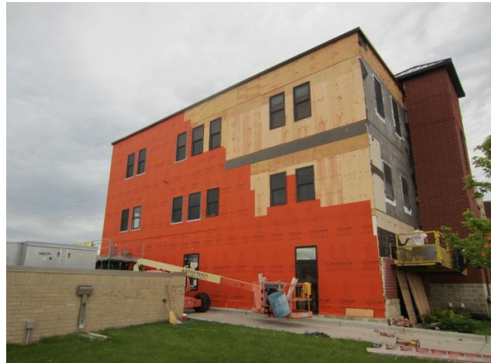
Over 32,000 sq. ft. of WrapShield SA Self-Adhered was installed on Woodhaven Plaza.
