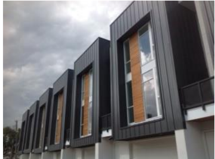
Over 10,000 sq.ft. of RevealShield UV Stable Water Resistive Vapor Permeable Air Barrier Membrane was installed on the Willits Parcel 4C Town homes in Basalt, Colorado.
