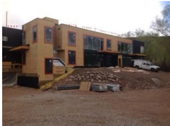
RevealFlashing Pre-Cut Flashing Membrane and VaproLiqui-Flash components were used to flash window and door rough openings.
