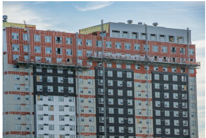
Over 110,000 sq. ft. of RevealShield SA Self-Adhered (black) and 120,000 sq. ft. of WrapShield SA Self-Adhered (orange) was installed on Washington Place in Tukwila, WA.
