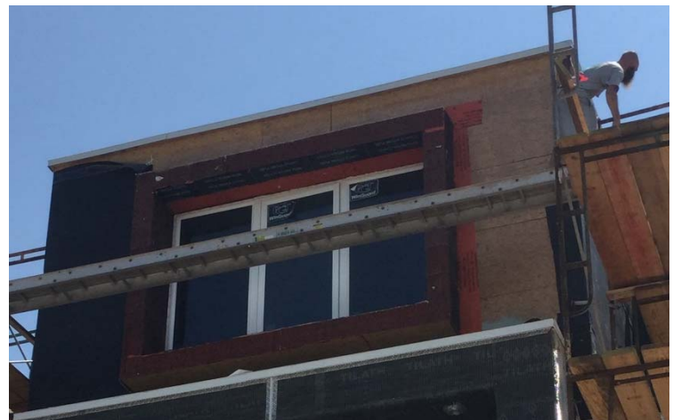
Upper window VaproFlashing SA Self-Adhered installed around the window, WrapShield RS Rain Screen 7mm (black/orange) installed as a field membrane provides an air cavity and drainage plane for the stucco façade helping to reduce the incidence of moisture related damage.
