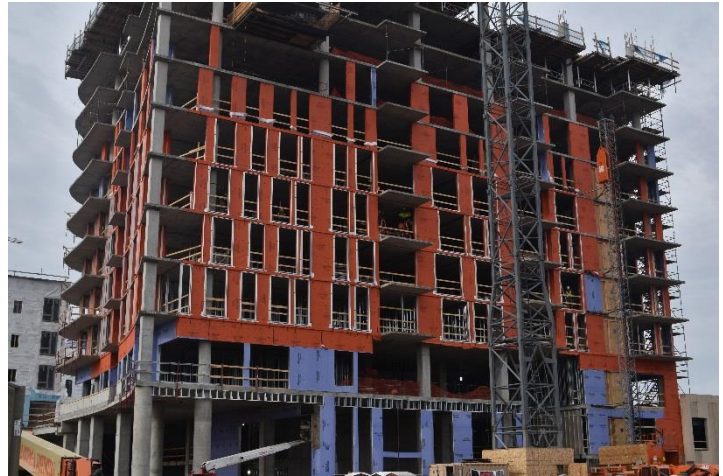
WrapShield SA Self-Adhered WRB/Air Barrier (orange) being installed on NordHaus urban development community in Minneapolis, MN.
