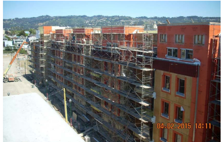
Over 330,000 sq. ft. of WrapShield RS Rain Screen with 7mm built-in drainage matrix was installed on Mural Apartments. The drainage matrix provided a cost-effective rain screen cavity behind the stucco and fiber cement lap siding.
