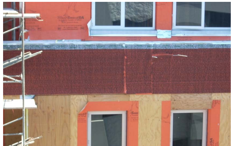
Along with the WrapShield RS Rain Screen field membrane, VaproFlashing SA Self-Adhered and VaproLiqui-Flash were applied on approximately 200 window openings, saving hundreds of labor hours compared to traditional flashing methods.
