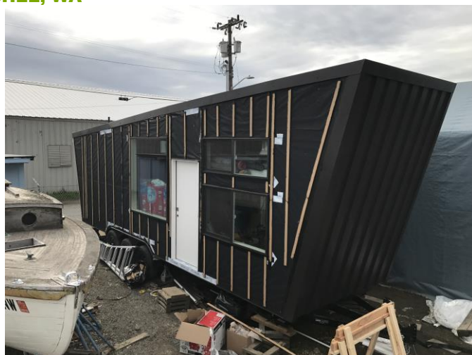
RevealShield SA Self-Adhered (black) was installed on 'Modern Wagon', a tiny house prototype in Wenatchee, WA.
