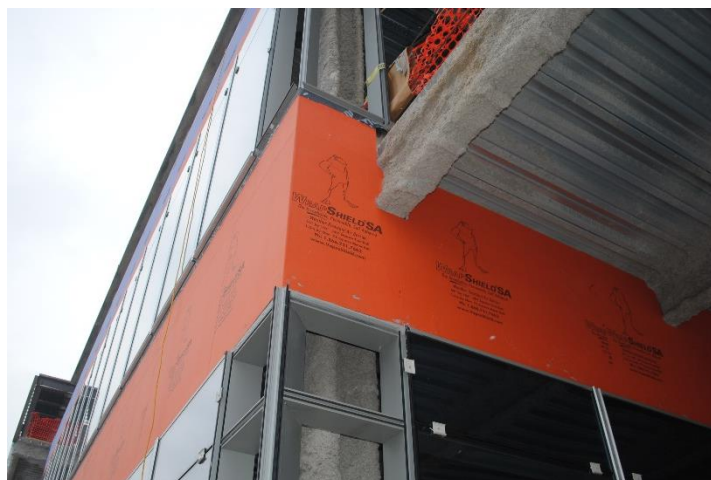
Over 190,000 sq. ft. of WrapShield SA Self-Adhered Water Resistive Vapor Permeable Air Barrier Sheet was installed on the JW Marriott, which is part of the $325 million Mall of America expansion project.
