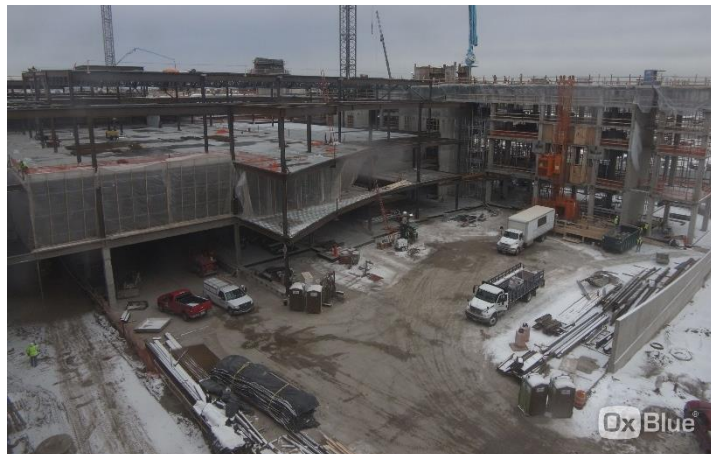
Stay up-to-date on the Mall of America hotel expansion project with views from the Mortenson Construction webcam: http://oxblue.com/open/mortenson/moa1c
