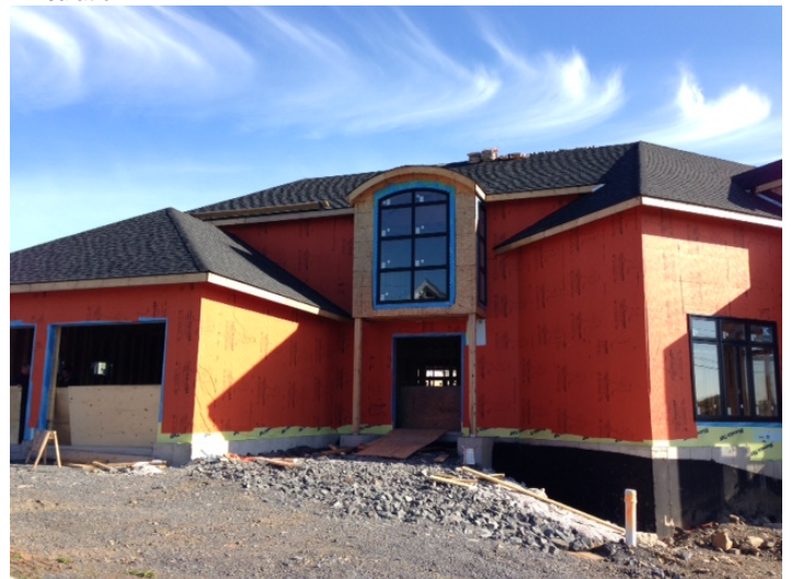
Over 1,500 sq.ft. of WrapShield Water Resistive Vapor Permeable Air Barrier Sheet was installed over OSB.
