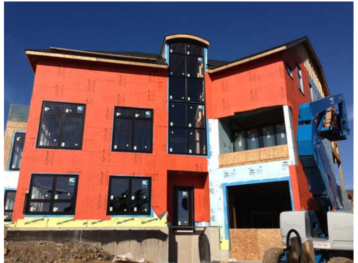
Over 6,000 sq.ft. of WrapShield SA Self-Adhered Water Resistive Vapor Permeable Air Barrier Sheet was installed over the XPS rigid insulation.
