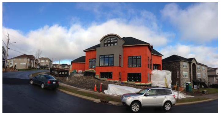
The homeowner chose VaproShield products to create a vapor permeable, breathable air barrier, which minimizes air leakage and reduces energy costs for the life of the residence.
