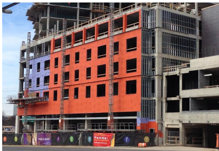
Over 100,000 sq. ft. of WrapShield SA Self-Adhered Water Resistive Vapor Permeable Air Barrier Sheet was installed at Mid Pike Block 10 in Rockville, MD.
