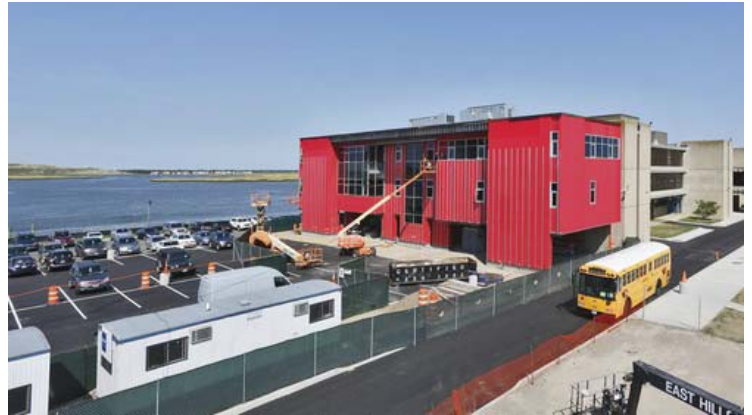
Over 50,000 sq. ft. of WrapShield SA Self-Adhered air barrier installed on the $16.5 million dollar addition to Long Beach High School in Long Island, New York.
