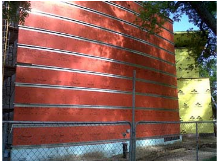
WrapShield SA Self-Adhered was installed over DenGlas sheathing, behind baffle-jointed metal panel system.
