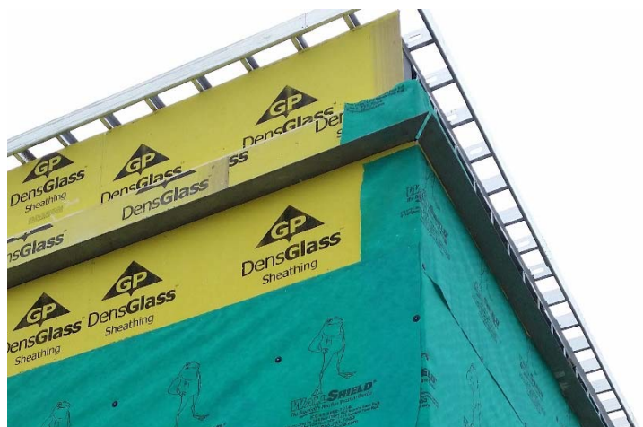
Approximately 8,000 sq. ft. of WallShield Water-Resistive Barrier Membrane was installed over Dens Glas ® Sheathing.
