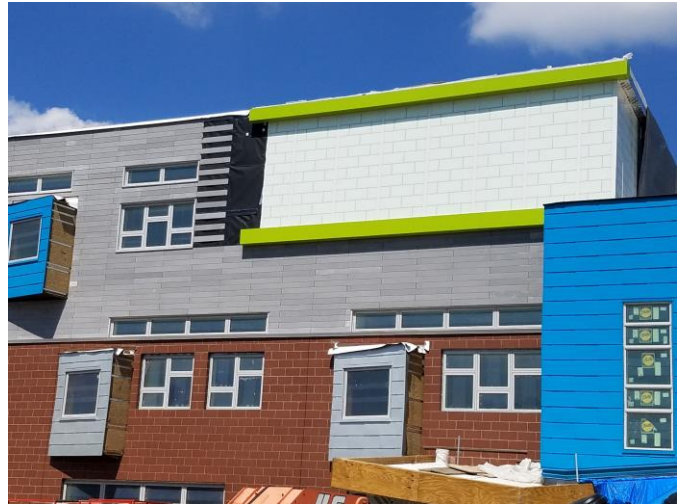
60,000 sq. ft. of RevealShield IT Integrated Tape (black) was installed behind UHPC (ultra high performance concrete) panels
