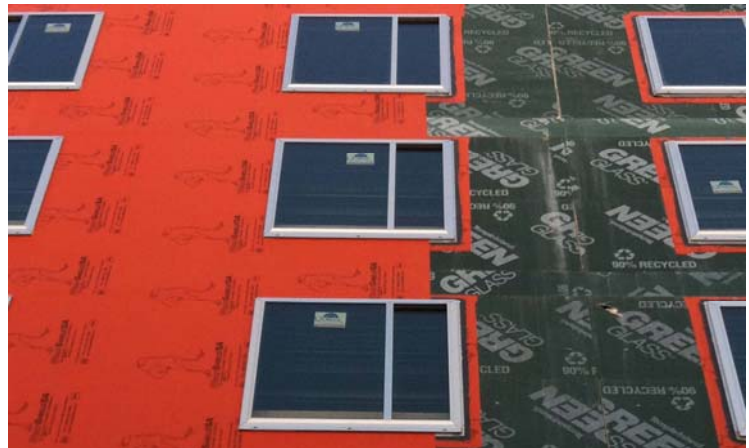
The energy-efficient envelope of Hyatt Place Chicago – South/University Medical Center decreases energy costs by 20% over a standard facility of similar size.
