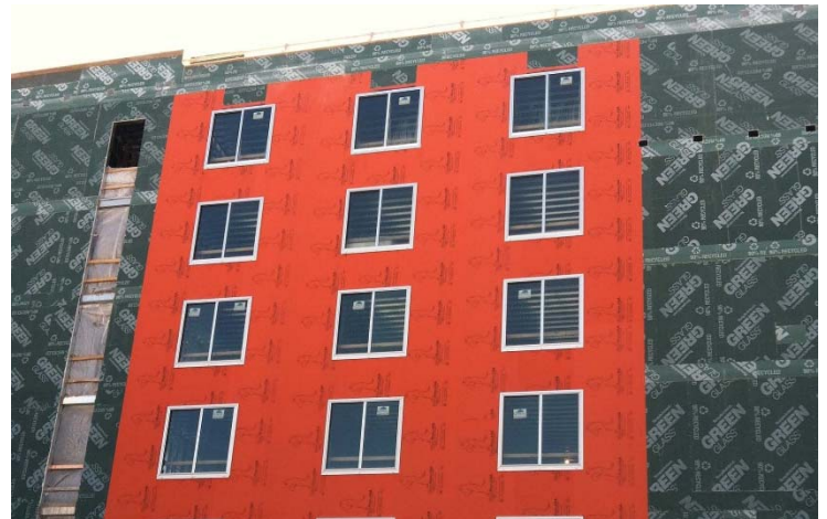
Over 54,600 sq. ft. of WrapShield SA Self-Adhered Water Resistive Vapor Permeable Air Barrier Sheet was installed at Hyatt Place Chicago – South/University Medical Center in Chicago, IL.
