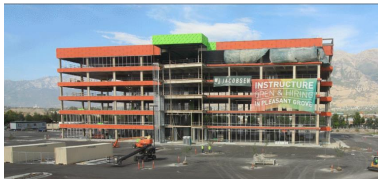
WrapShield SA Self-Adhered WRB/Air Barrier (orange) installed on Grove Tower in Pleasant Grove, UT.
