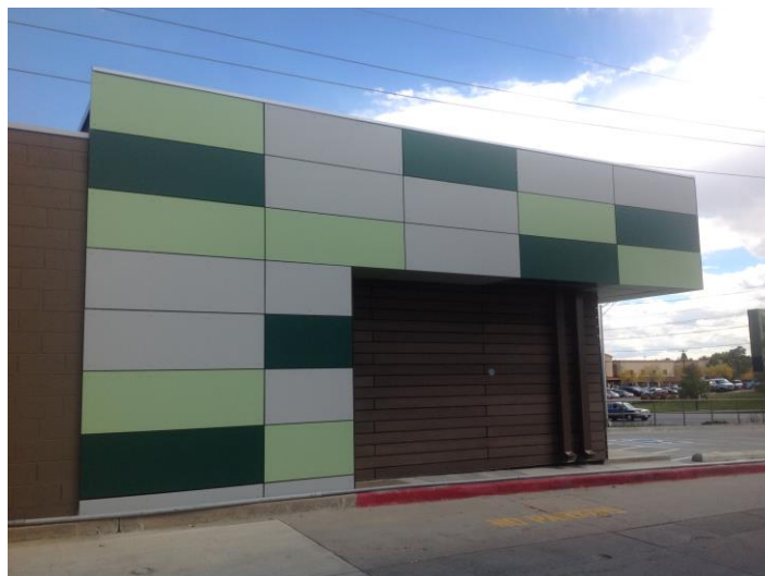
Over 4,000 sq.ft. of RevealShield SA Self-Adhered was installed on the Green Man building.
