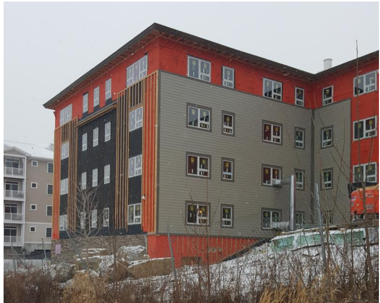
RevealShield SA Self-Adhered (black) was installed behind open-joint cladding on the Residence at Quarry Hill assisted living center in Burlington, Vermont.
