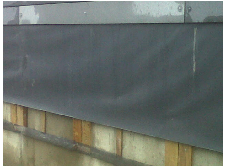
A single layer of RevealShield Black, UV Stable Water Resistive Vapor Permeable Air Barrier Membrane is installed on this private residence in Vancouver, British Columbia.
