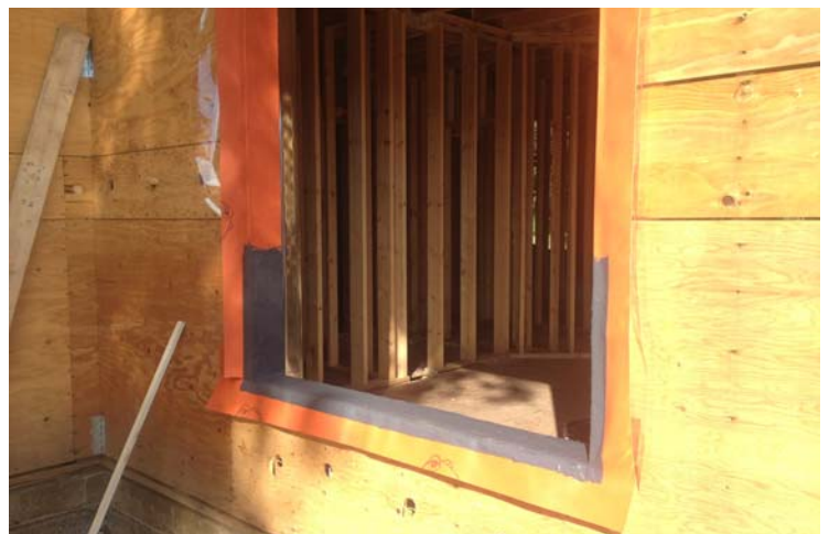
(above) VaproLiqui-Flash (gray) liquid applied waterproof flashing material is applied around the rough opening of a window.
