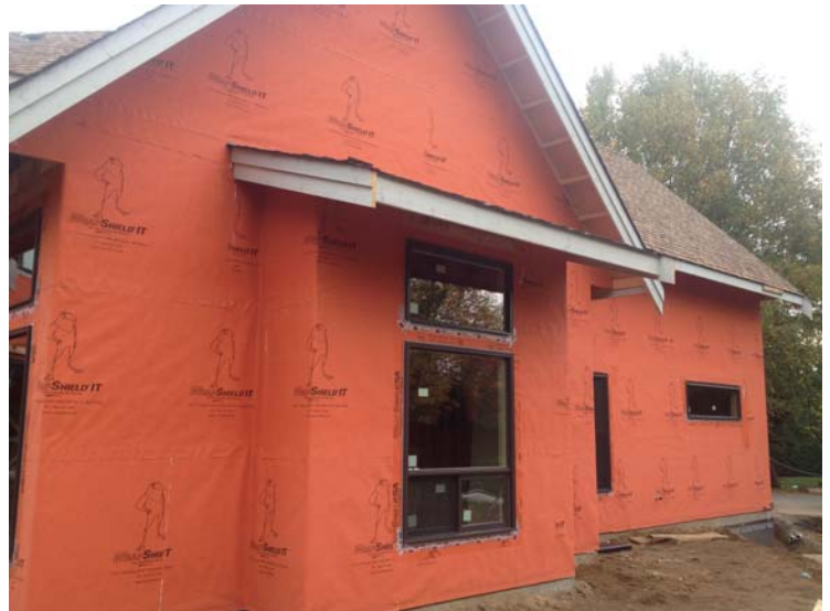
Over 4,000 sq. ft. (1,219 M 2 ) of WrapShield and WrapShield SA Self-Adhered Air Barrier is installed on a private residence in Langley, British Columbia.
