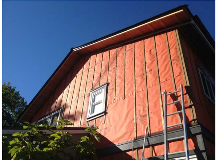
Over 3,000 sq. ft. (278 M 2 ) of WrapShield and WrapShield SA Self-Adhered Air Barrier is installed as a retrofit on a private residence in Burnaby, British Columbia.
