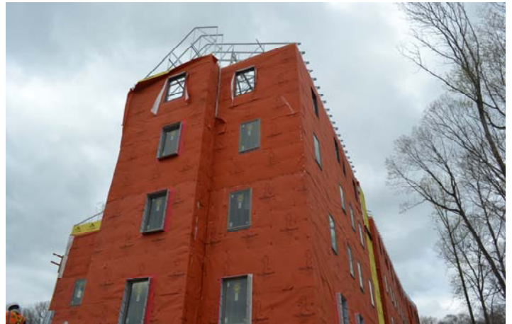
Over 120,000 sq. ft. of WrapShield Water Resistive Vapor Permeable Air Barrier Membrane was installed on Princeton University's Lakeside Graduate Housing complex.
