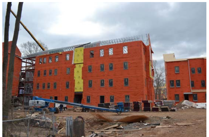
With zero VOC's WrapShield contributes LEED points towards the Lakeside Graduate Housing complex's goal of LEED silver certification.
