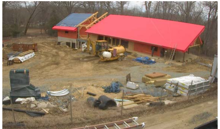
Approximately 2,800 sq. ft. of WrapShield SA Self-Adhered Water Resistive Vapor Permeable Air Barrier Sheet (orange) and 4,650 sq. ft. of SlopeShield SA Self-Adhered Water Resistive Roof Underlayment Sheet (red) was installed on the Alice Ferguson Foundation's Potomac Watershed Study Center.
