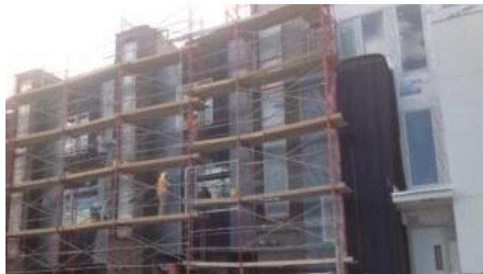
Over 15,000 sq. ft. of RevealShield UV Stable Water Resistive Vapor Permeable Air Barrier Membrane was installed on Durant Condominiums in Aspen, Colorado.
