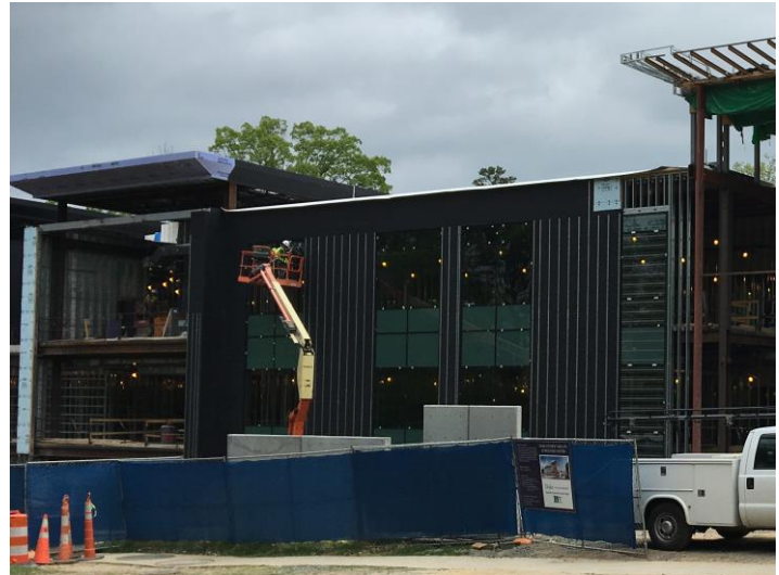
RevealShield SA Self-Adhered (black) was installed on the Student Health and Wellness Center at Duke University.
