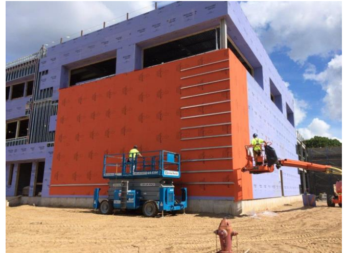
60,000 sq. ft. of WrapShield SA Self-Adhered Water Resistive Vapor Permeable Air Barrier Membrane was installed at CREC Academy of Aerospace and Engineering in Windsor, CT.
