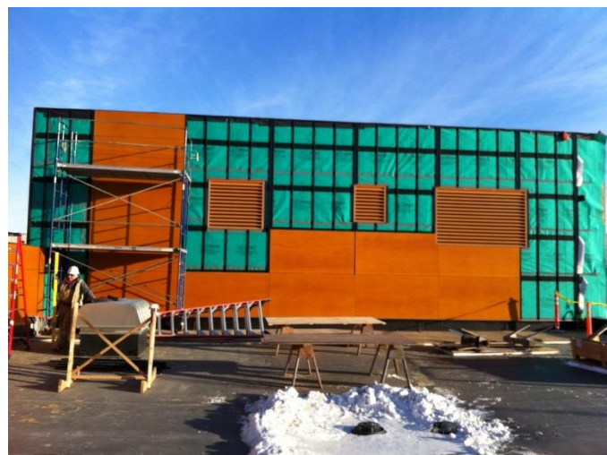
Over 20,000 sq. ft. of WallShield Water Resistive Barrier Sheet was installed on the Covenant House in Alaska.
