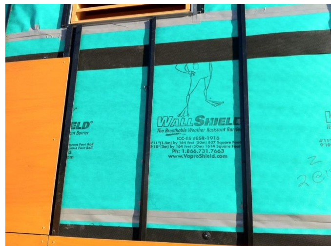
Strips of WrapShield Black Water Resistive Vapor Permeable Air Barrier Membrane was used at the open joints.
