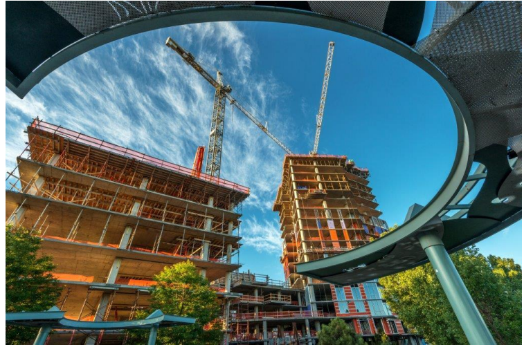
WrapShield SA Self-Adhered WRB/Air Barrier (orange) is being installed on The Confluence in Denver, Colorado.
