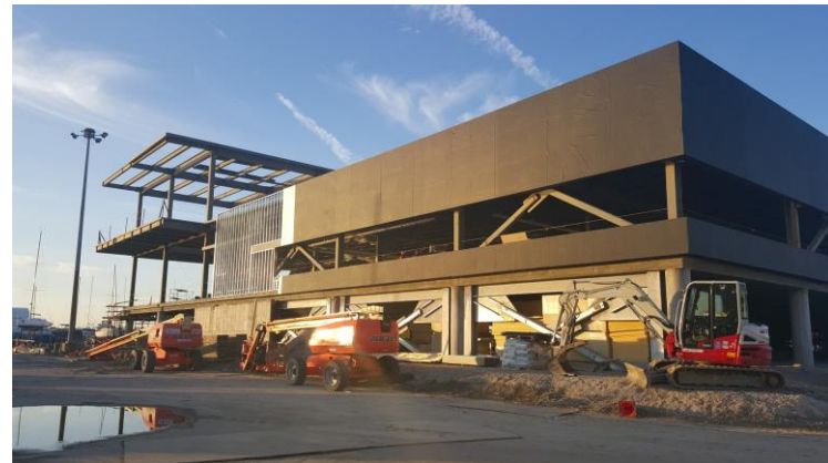
RevealShield SA Self-Adhered was installed over Thermax™ sheathing and behind open joint metal panel cladding.
