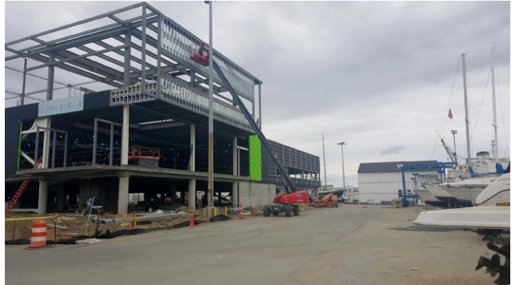
Over 20,000 sq.ft. of RevealShield SA Self-Adhered was installed on the Zucker Graduate Center at Clemson University Restoration Institute.
