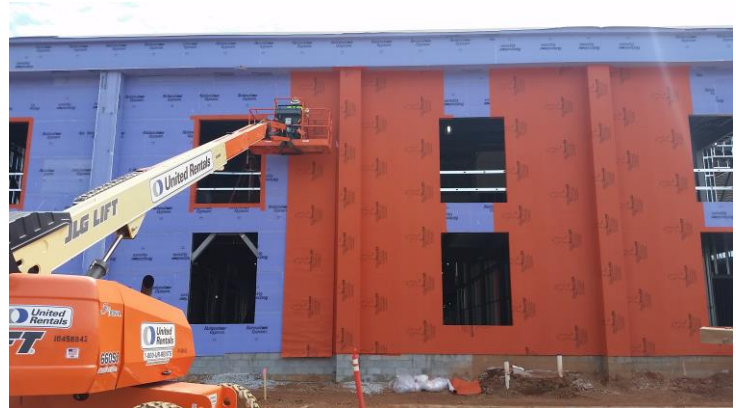
WrapShield SA Self-Adhered (orange) was installed over gypsum sheathing on the new Clemson University Football Operations Center in Clemson, SC.
