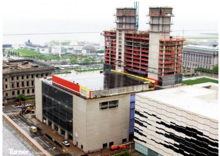
Hilton Cleveland Convention Center Hotel relied on WrapShield SA Self-Adhered (orange) to ensure a smooth, cold weather construction and superior building longevity.
