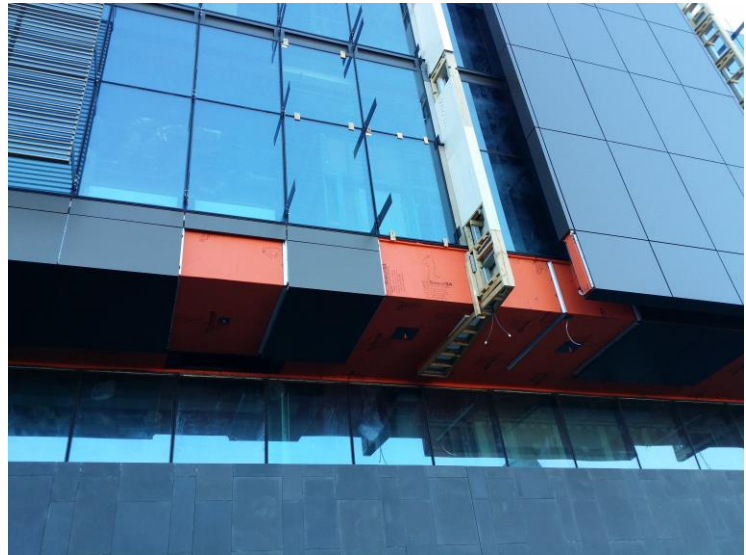
WrapShield SA Self-Adhered (orange) was installed behind cladding on the Christchurch Justice & Emergency Services Precinct in Christchurch, New Zealand.
