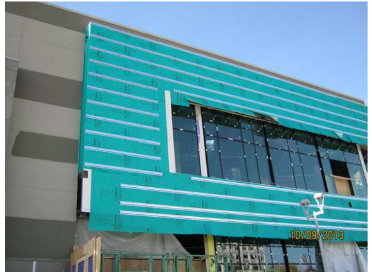
Approximately 4,000 sq. ft. of WallShield and 1,000 sq. ft. of RevealShield was installed on Double Zero Pizza in Calgary, Alberta.
